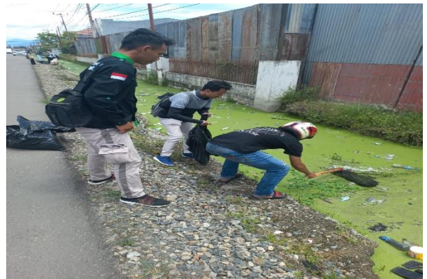
Figure 13. Drainage cleaning from plastic waste (Source: Personal Documentation, 2022)
